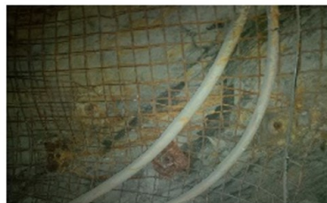
Severe damage or corrosion of mesh, rock bolts, and other equipment from leaching and oxidation in reactive ground. Oxidation of the actual rock is also visible behind the mesh. These may be used as indicators to reactive ground conditions.
