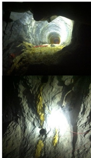
These images show reacting sulphides and explosive leaking from the drill hole during the Q356 incident. It displays a rich yellow colour.
