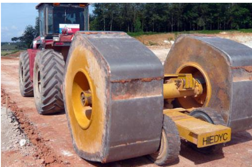
Figure 3. 5-sided RDC module (Infratech).
